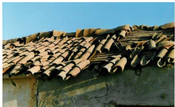
Building Construction. Fig. 13 Country tile roof (Gujarat, India). Split bamboo placed close together serves as battens (photo by the author).
